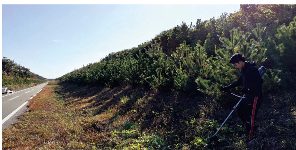
Maintaining sea embankment and disaster prevention forests on the Enshu Sea coast
